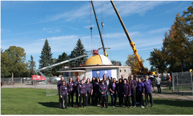
On September 22, crews began installing a new concrete dome onto, an important historical city landmark, the 59-year-old Queen Elizabeth Planetarium. Science centre staff gathered to celebrate the occasion.
